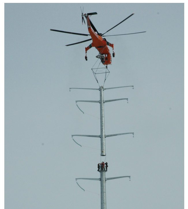
A helicopter hoisted transmission tower pieces for the construction of the Monticello-to-St. Cloud CapX2020 project.
