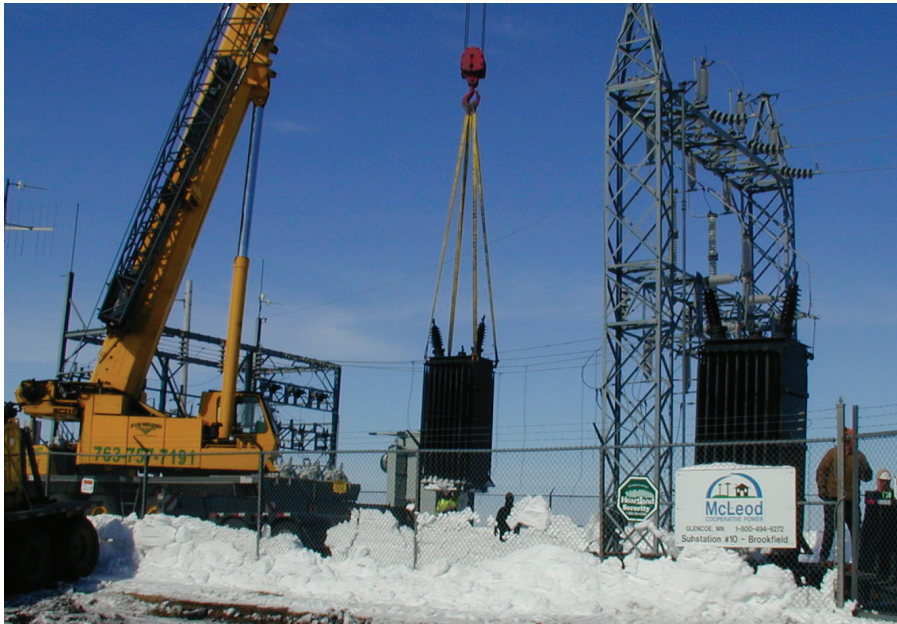
A crane lifts one of the 833-kVa transformers out of the Brookfield Substation and onto a waiting trailer.
