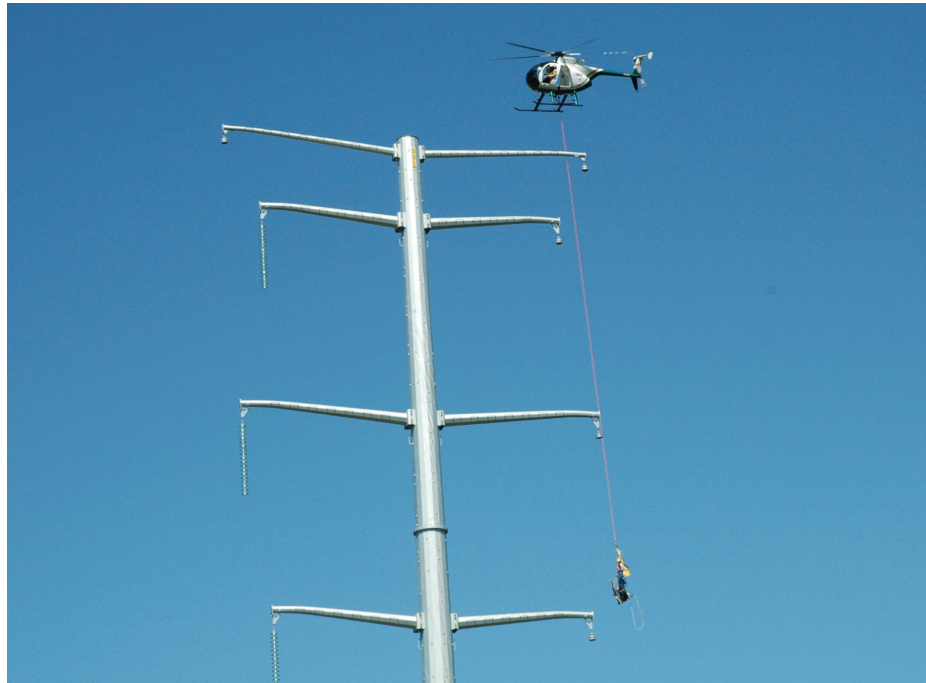
Workers from Air 2 attach pulleys that will be used to string conductor between towers. Helicopter installation is faster and more efficient than using ground-based cranes in this area.
