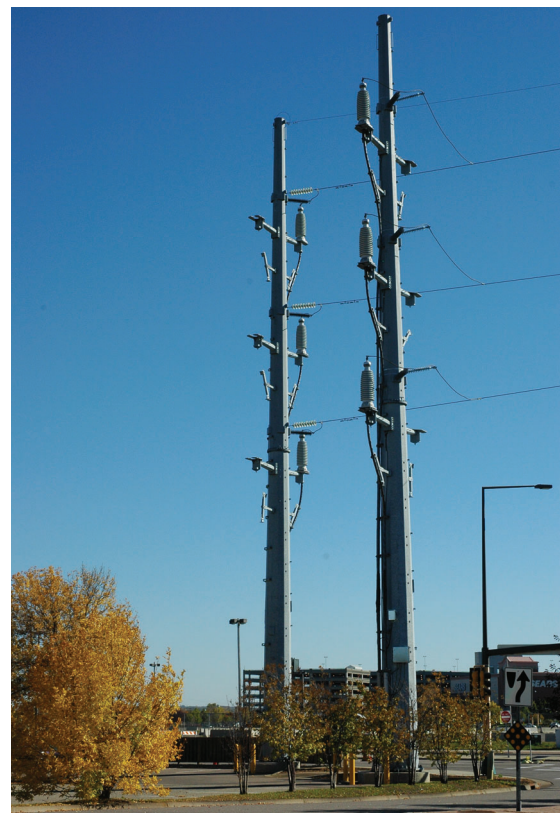
Riser structures are required in some areas when burying transmission lines underground.
