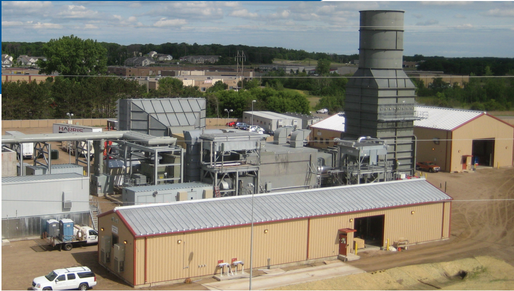
Elk River Peaking Station, Elk River, Minn., Sherburne County
