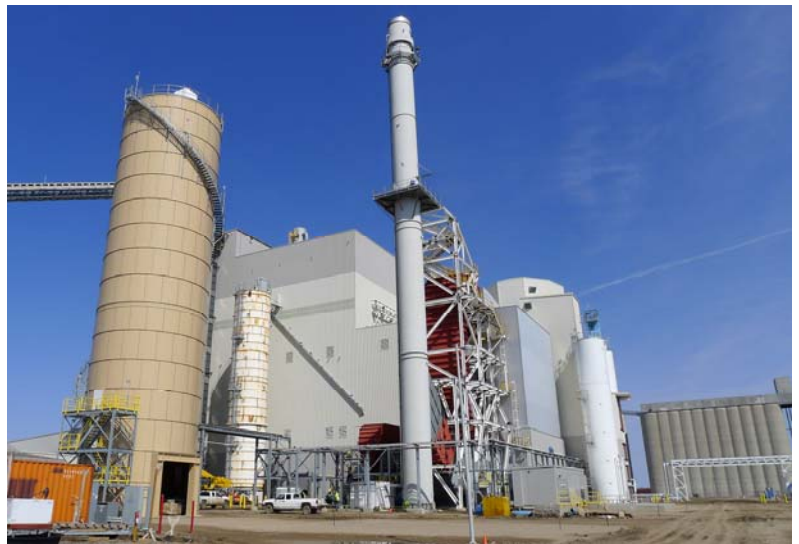
As a combined heat and power plant, Spiritwood Station will generate electricity and steam.
